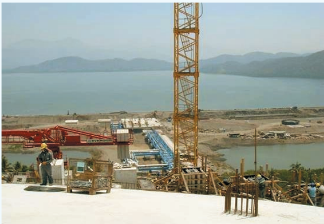
Jetty Platform at the Manzanillo LNG Terminal in development Source: Mitsui & Co.,
